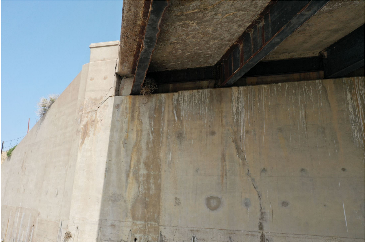
Picture 3 – Corrosion, cracking, efflorescence
